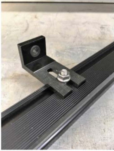
Figure B3e. #CMP-KT connected to Mounting Systems racking system
