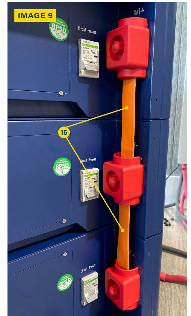
16 PARALLEL BATTERY CABLE
