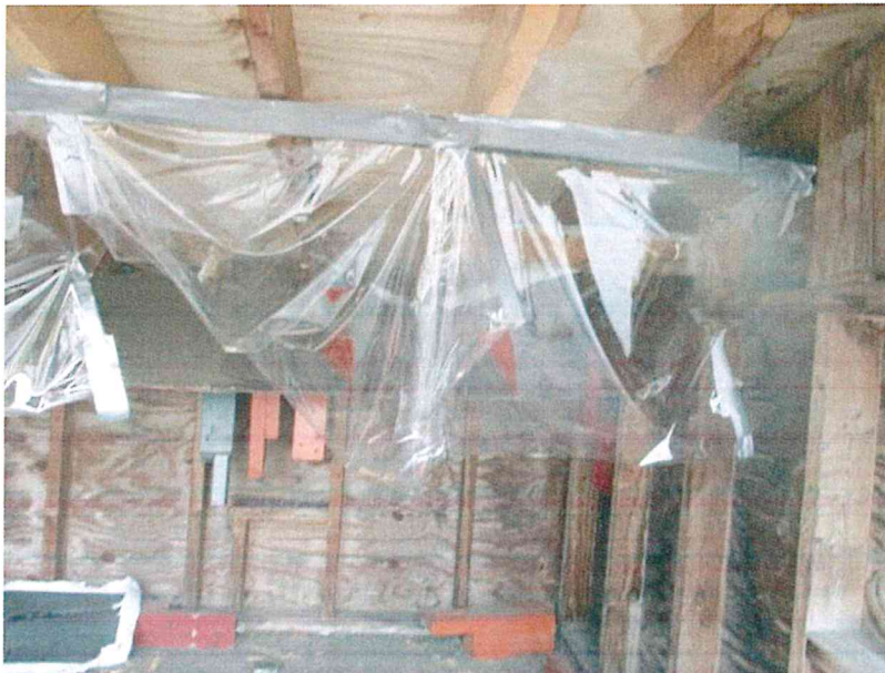
Photo No. 10 Underside of Test Specimens #3 and #4 After Testing
